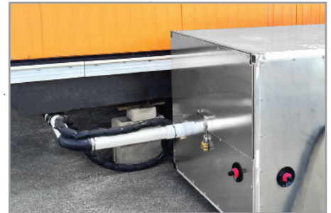
View of an installed Water System
