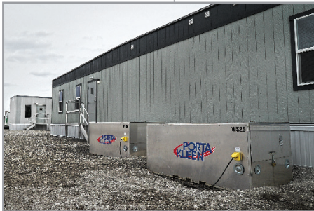
Several installed Water Systems
