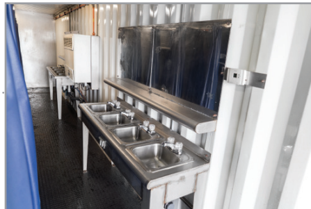
View of the sinks, mirror, and shelf
